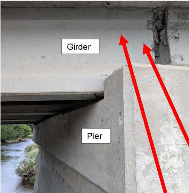
Photograph of Structure 013-092 Shear Cracks (Typical of all girders)
